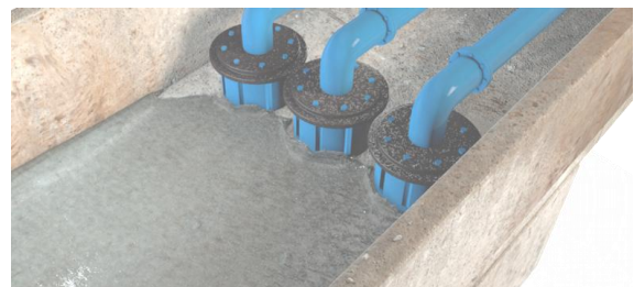
Figure 2: Parallel arrangement of hydrocyclones in the hydroelectric diversion channel.
