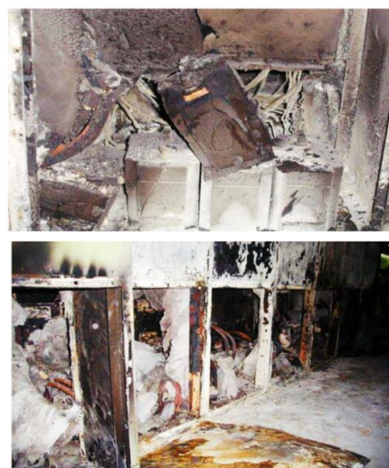
Figure 1: Damage to the voltage transformer.
