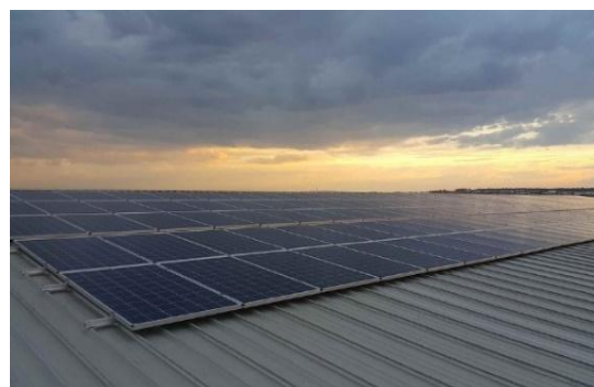
Figure 3: Solar panels operating in shaded conditions.
