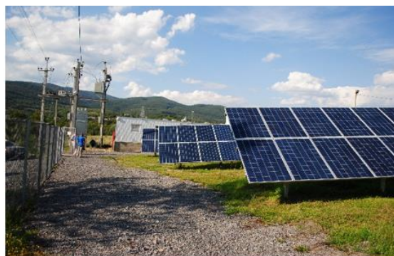
Figure 1: Solar power plant complex.
